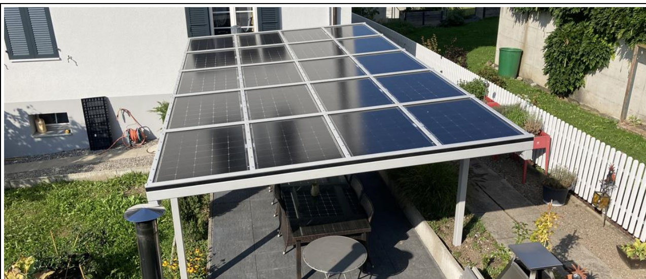
PVA 3S Swiss Solar Solutions – TeraSlate – 4kWp – Indach Pergola – Steffisburg - 2024
